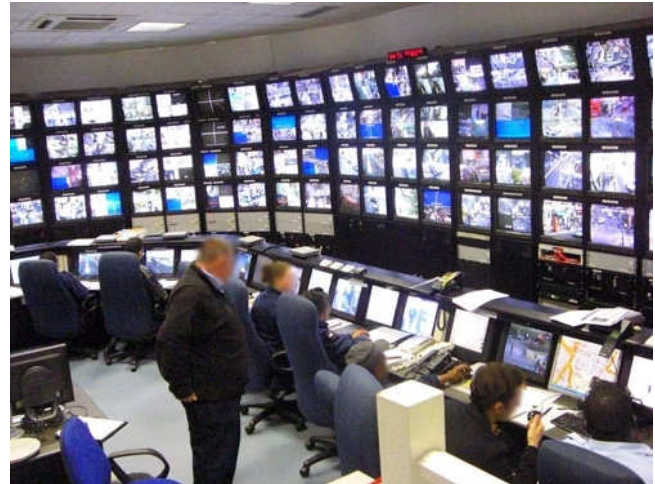
Figure 1: CCTV control room, site UK3
